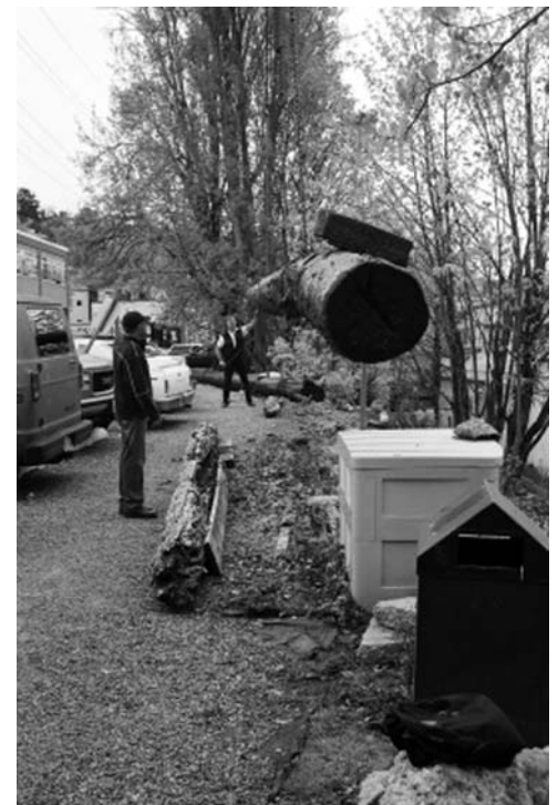
Volunteer Christian Lint steadies a huge log, assisted by a Northern Marine Salvage and Development crew member.
