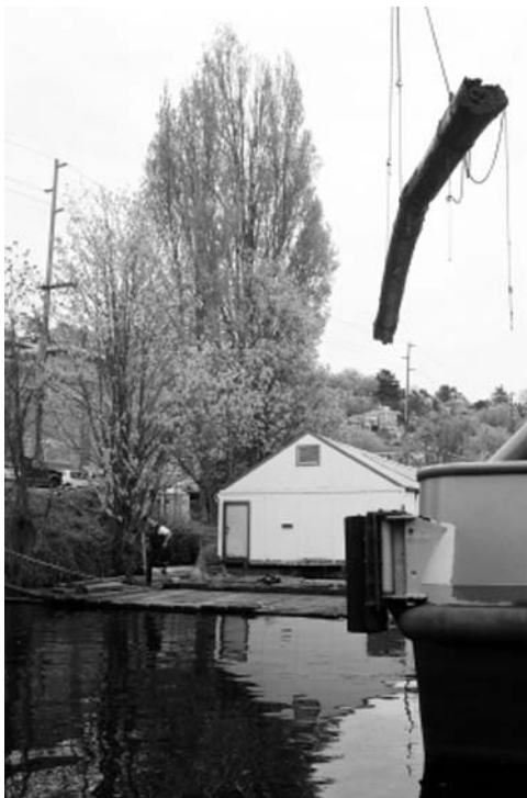
Spliced together from an old dock, cedar logs are lifted over the trees.
