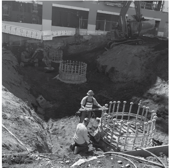
Workers on the Fairview Bridge project prepare support structures for the new bridge.
