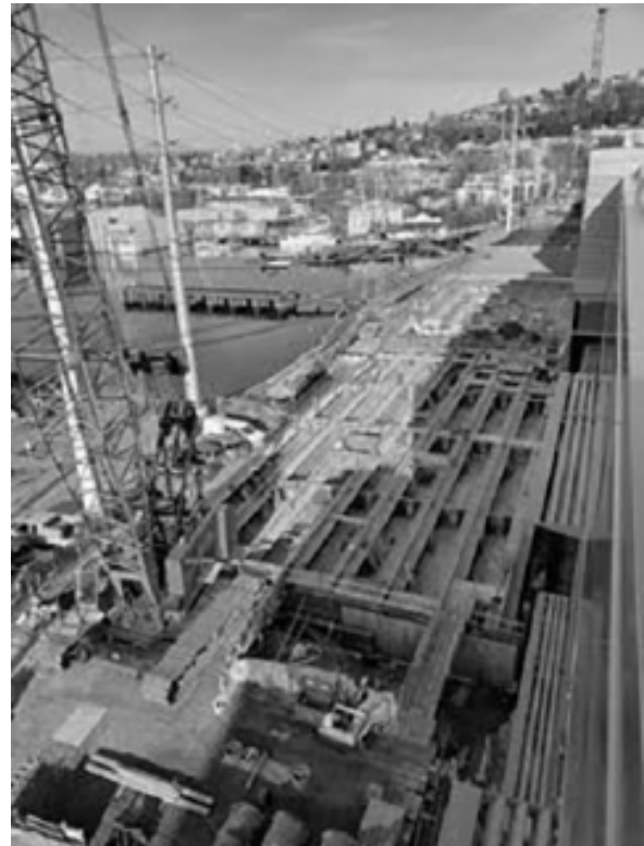
A view from above of the continuing work in the Fairview Avenue North bridge. Crews were beginning to pour concrete for the bridge surface. Seattle Department of Transportation Photo
